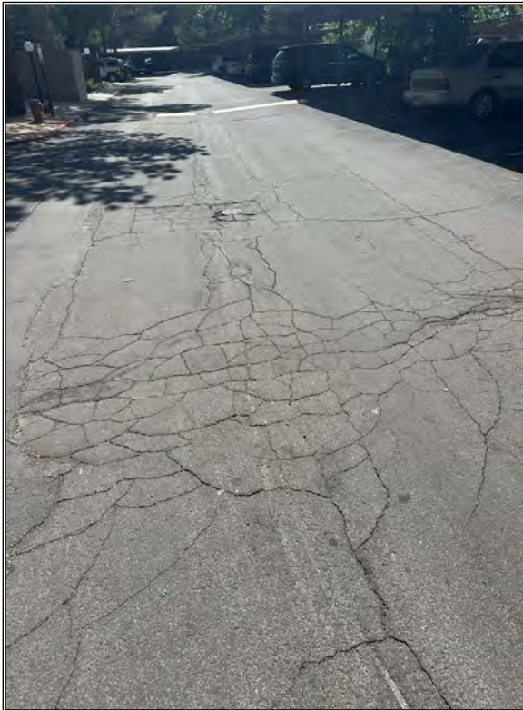
IMAGE 1: Alligator Cracking at HA-02
